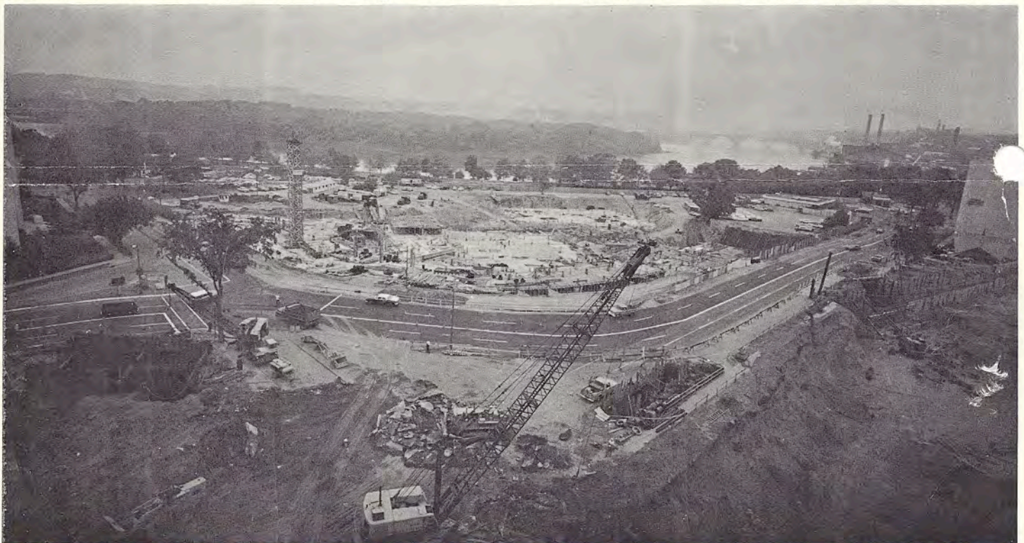
The Watergate site in August, 1964, looking from the East to the main entrance of Watergate East. Construction began in February, 1964, and is scheduled for completion this fall.
